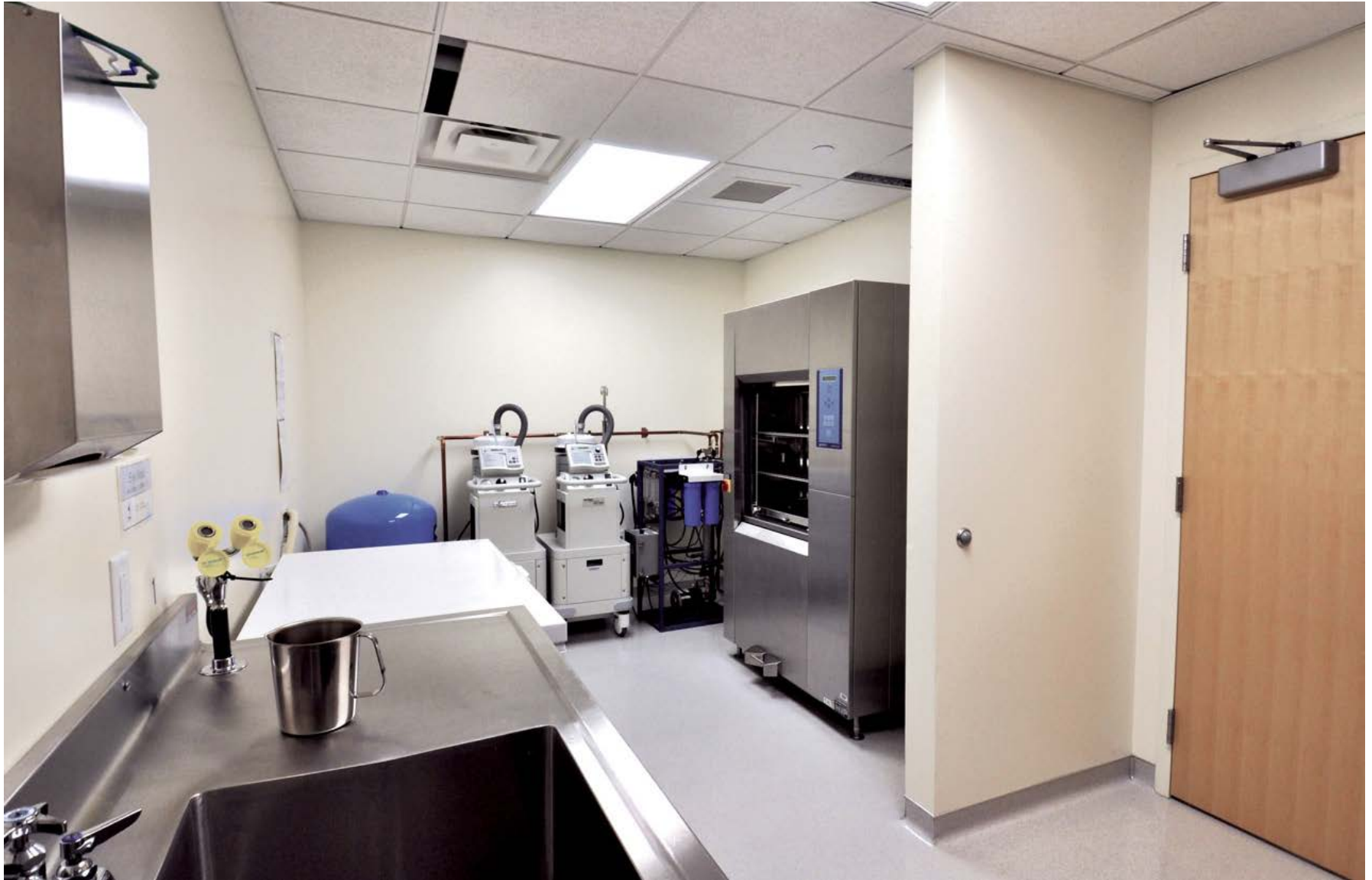
Fully functioning instrumentation and equipment decontamination space within the lab. Featuring a hand wash sink station for delicate surgical equipment and a full-size surgical instrumentation washer/disinfector.
